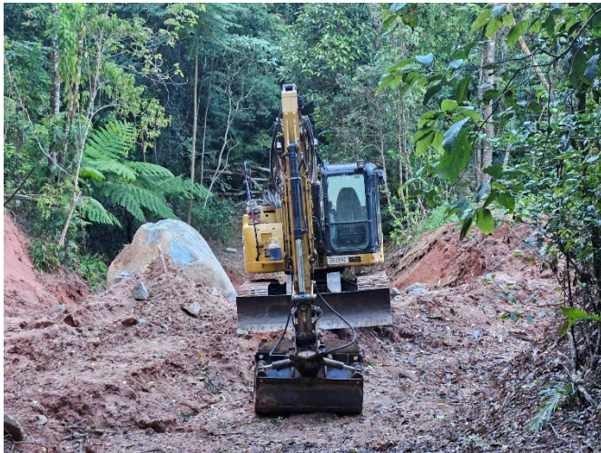
Wash-out on Bridle Creek Road. Photograph by Chrissy Warman
